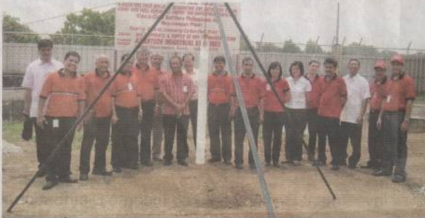
Coca-Cola Bottlers Philippines, Inc. (CCBPI) employees inaugurate the construction of a steam-boiler which uses rice hull or ipa to produce energy for its Meycauayan Plant. Operational since January 2009, the other plants of the Company will eventually utilize this technology.
